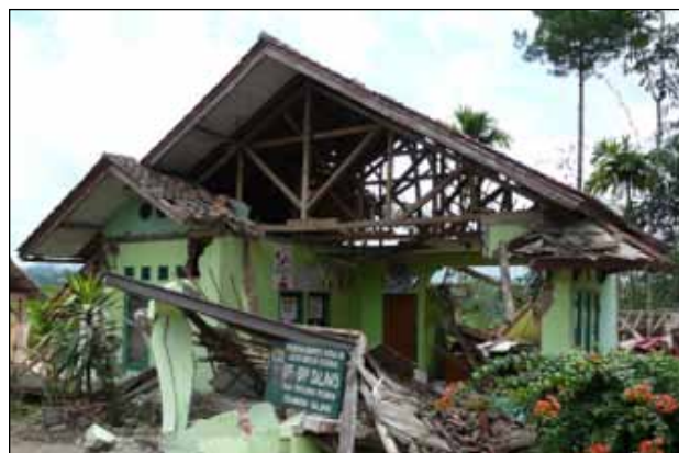
Figure 2. A building with confined masonry walls failed due to low-quality materials and poor workmanship.
